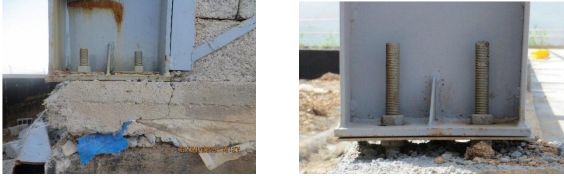
FIGURE 19. Gap Under Base Plates Casted with Floor
