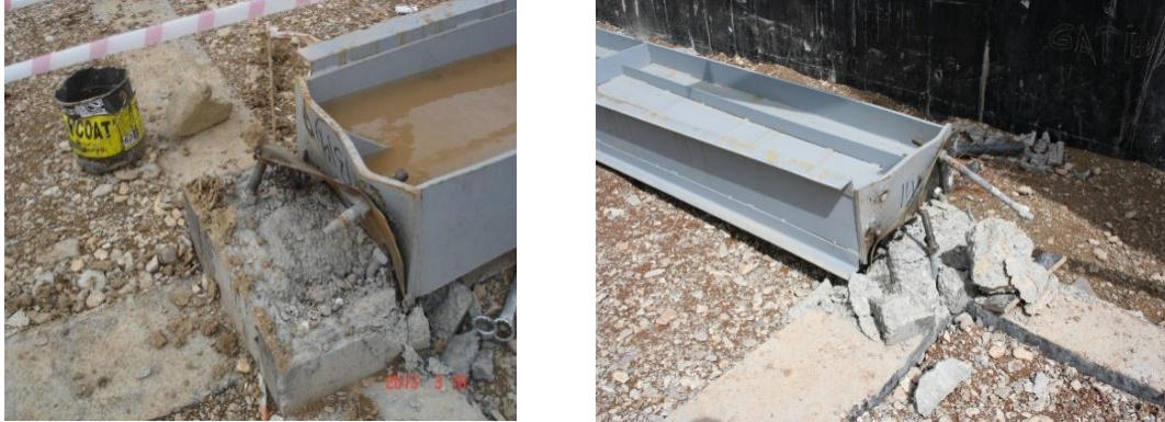
FIGURE 14. Anchor Rod Failure, Ductile Failure (left) and Non-Ductile Failure (right)
