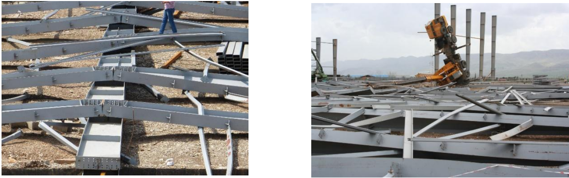
FIGURE 1. Collapsed Frame as Domino Action
