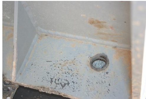
FIGURE 16. Base Plate Tear Through Failure
